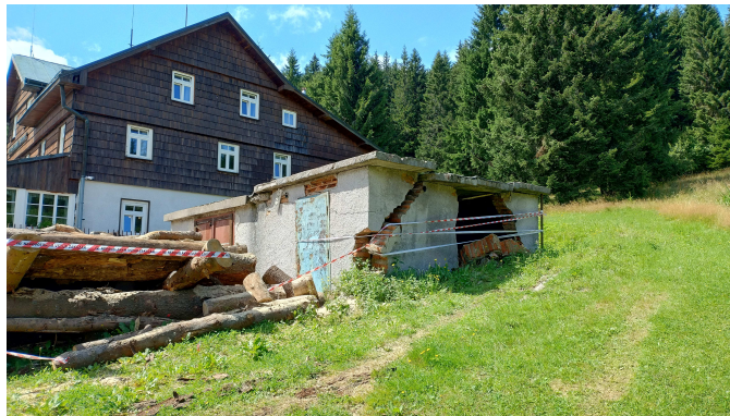
frost heave damaging constructions
