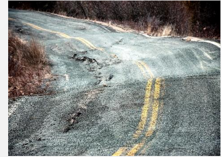
Permafrost damaged roads, Yellowknife, Northwest territories. Credit: Ryerson Clark/iStock
